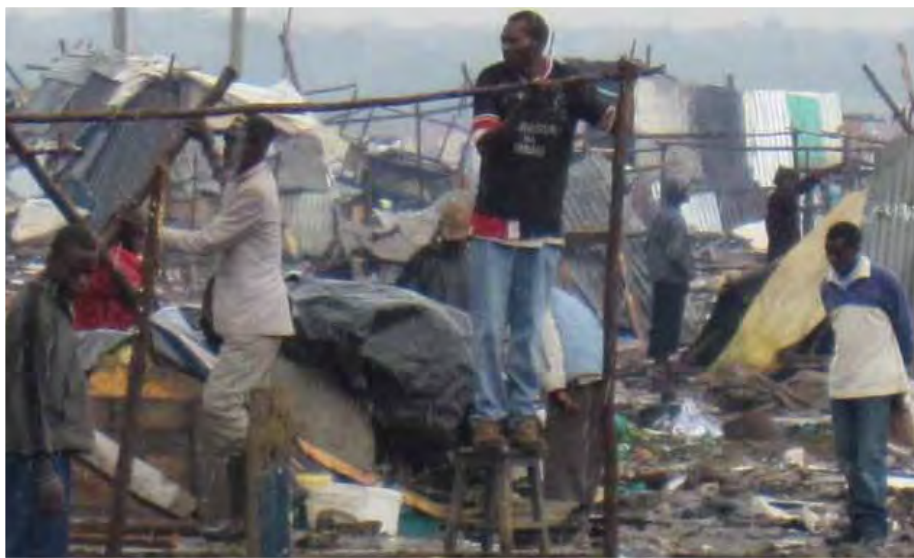
Communities reconstruct shelters after the Mitumba demolition in November 2011 © Save the Children, 2011
