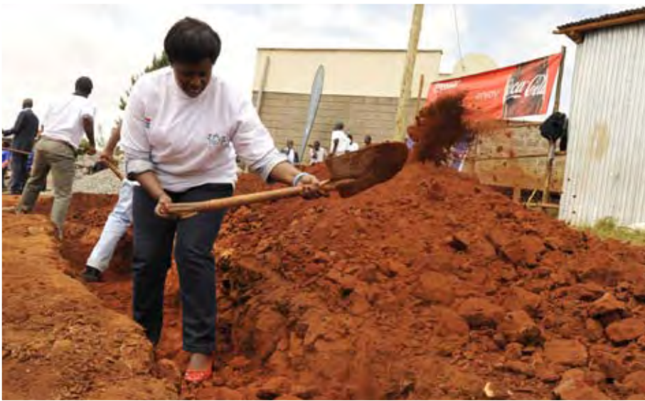
UNIC Administrative Assistant Janice Mbugua during the digging of the foundation for the classrooms at the HOYWIK Centre © UNIC, 2011
