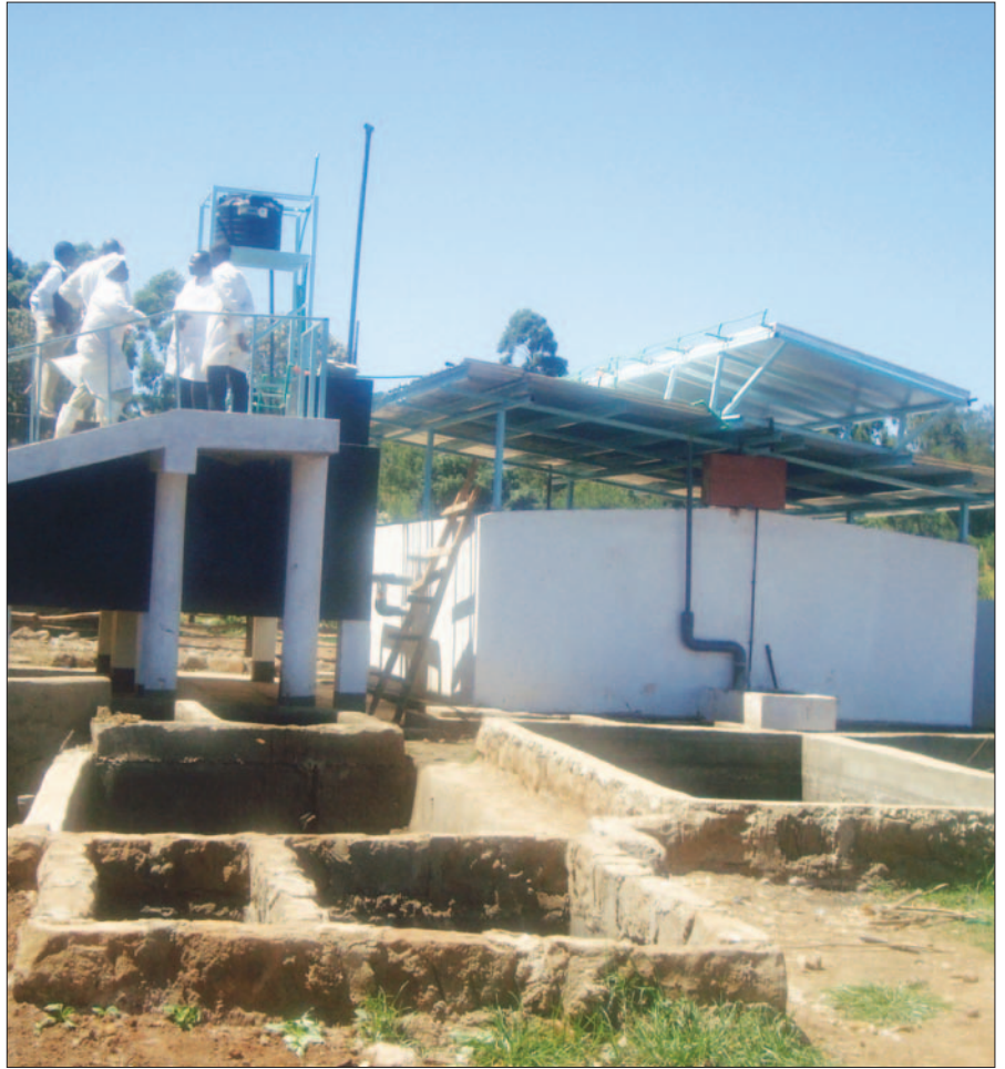
The Nyongara Biogas plant
